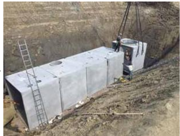
Stormceptor MAX installation. A ten box Stormceptor MAX unit was used to treat 110 ha. (5 boxes shown)
